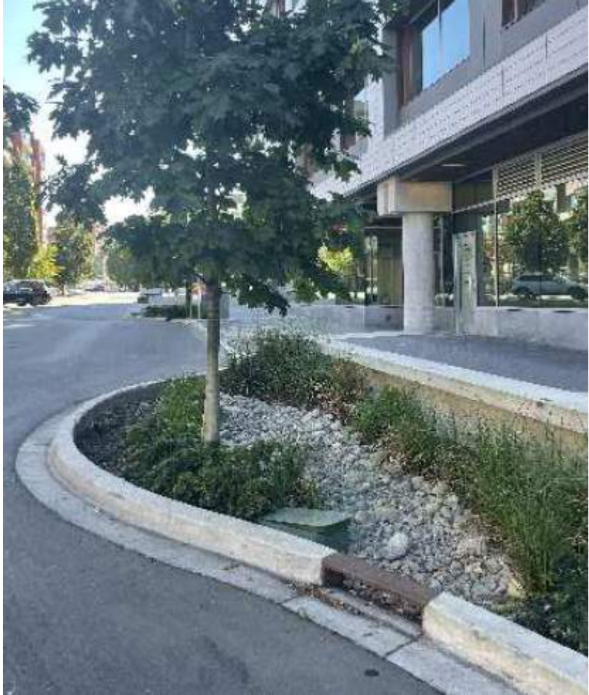
2. Street surface runoff collection into rain garden.
